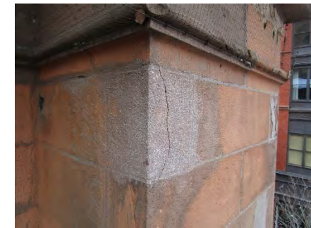
Deteriorated stone at pilaster corners require full stone replacement
