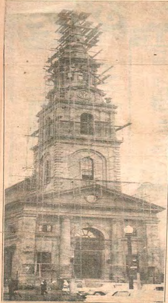
CHURCH'S NEW LOOK —The 100-year-old Arlington Street Church is getting a new look as workmen begin a $165,000 rejuvenating job on the Back Bay edifice. Scaffolding surrounds the steeple as they begin job of repointing and weatherproofing it. Exterior work is expected to be completed before Thanksgiving.
